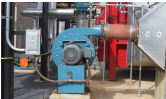
Top right: Main control panel mounted in control room. Remote panels located as needed.
